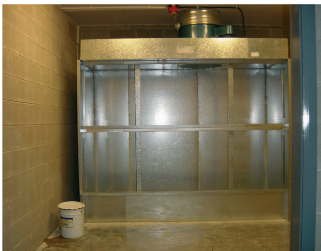
Photograph 5 Spray booth enclosure
