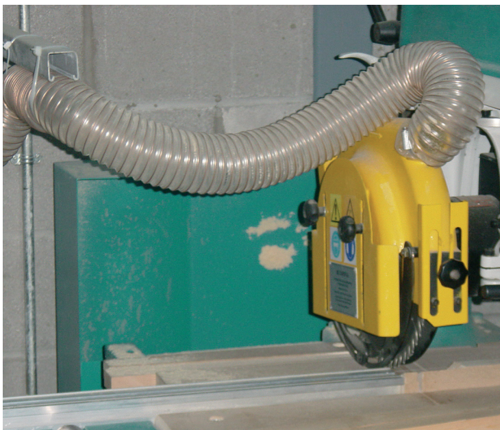
Photograph 6 Dust extraction system fitted to a cross-cut saw
